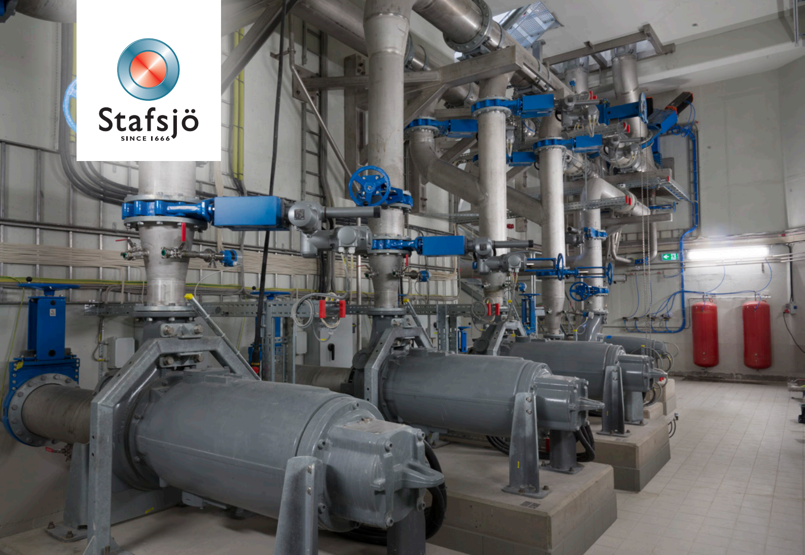
The pump station in the centre of Värnamo.
